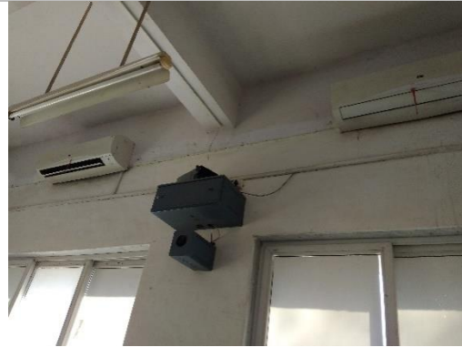
Lecture Capture Equipment and Air Conditioning
