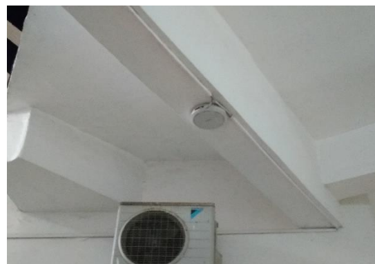
Wi-Fi – Router and AC
